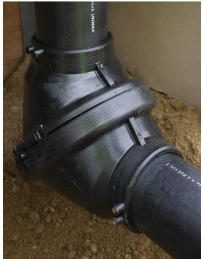
An installed 90 elbow.
