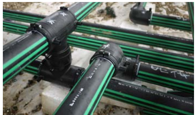
UPP 63mm suction and VR2 lines were also installed on site. Here two 63mm electrofusion tees are used to create VR2 branch lines.
