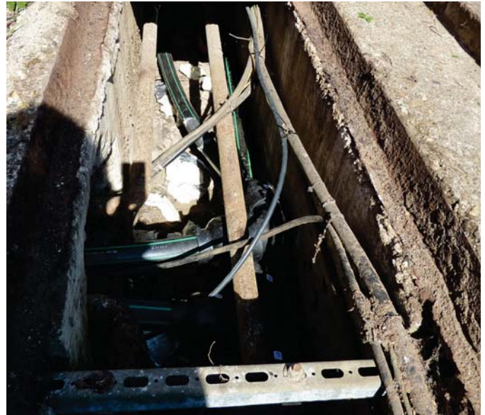
Existing steel fuel lines sitting next to new UPP Polyethylene lines in ducts during installation. Note the steel lines were removed once the new lines were completed and commissioned.
