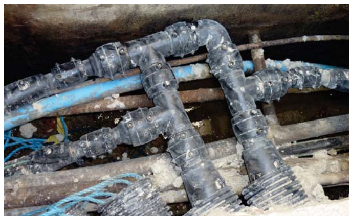
50mm (1.5") diameter UPP double wall ring main line protrudes and returns through ducts at the bottom of the shot and manifolds off into three 32mm (1") double wall boiler/generator feed lines
