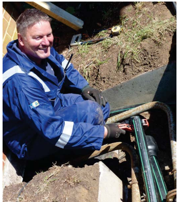
Experienced fuel installation engineer, Steve Picton of Adler and Allan completing work to the double wall UPP fuel lines
